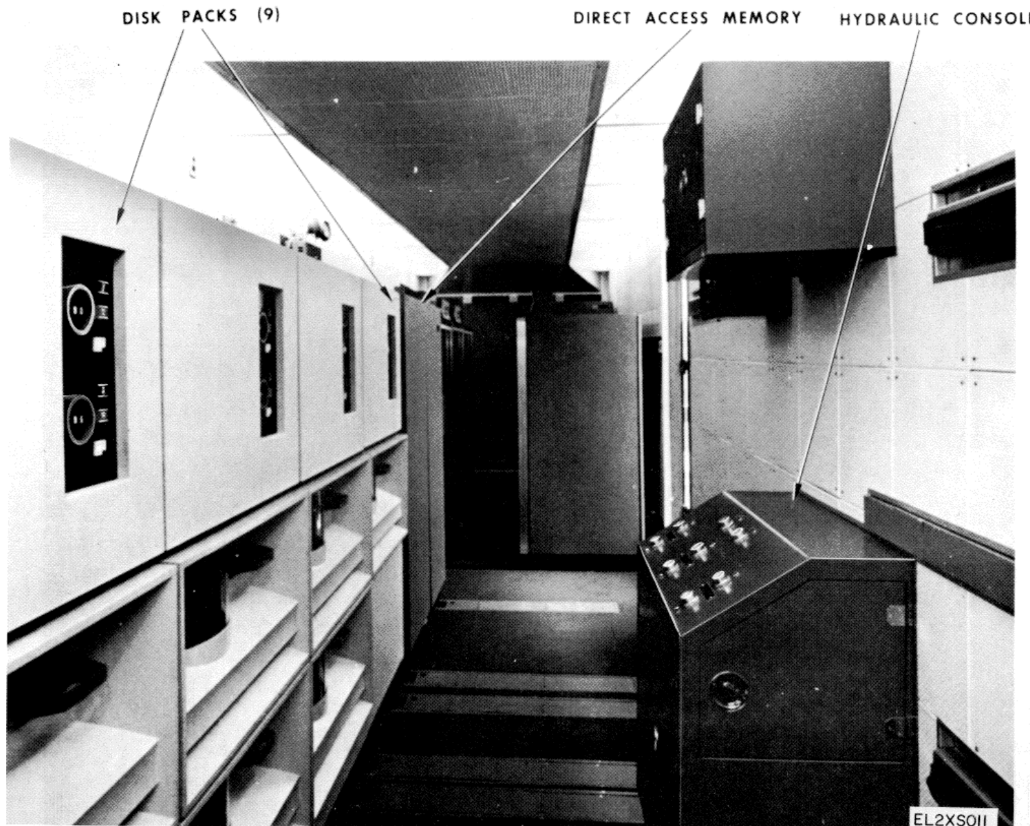
Figure 1-11. Data Storage Group OL-89(V)1 /MYK-8 (V), Interior Front View.
