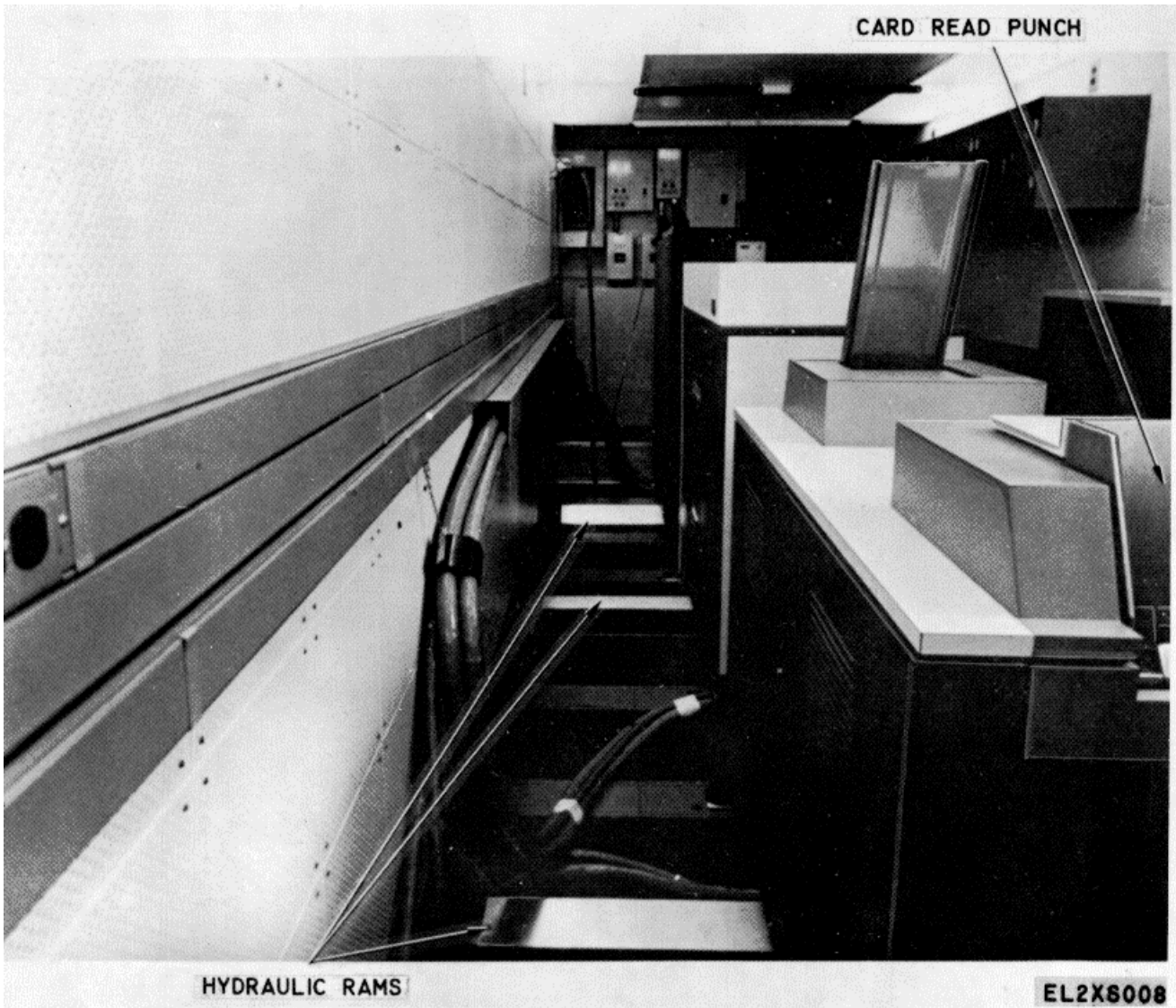
Figure 1-8. Data Analysis Central OL-88 (V) 1/MYK-8, Equipment Moved for Storage or Service.
